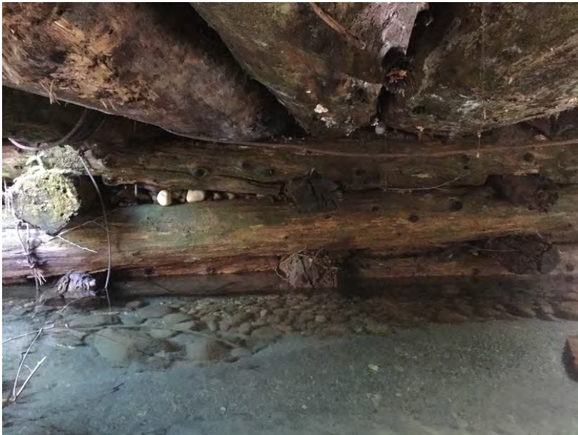
Top face log on left abutment cracked and settling
